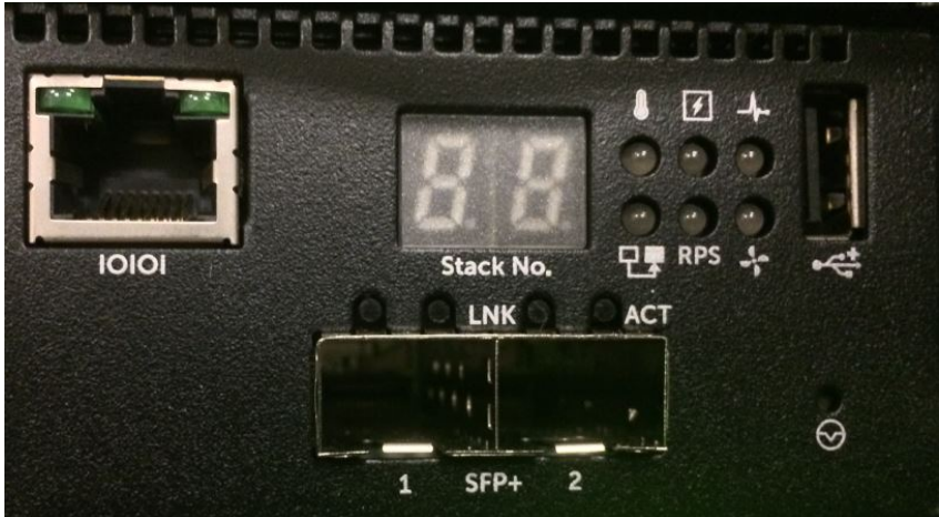
Figure 3-10. Dell EMC Networking N2024/N2048 Close-up
